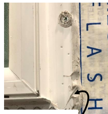
NAIL-FLANGE SET ON A BED OF CONTINUOUS SEALANT CREATES A WATERTIGHT JOINT. CONCEALED UNDER THE CLADDING
